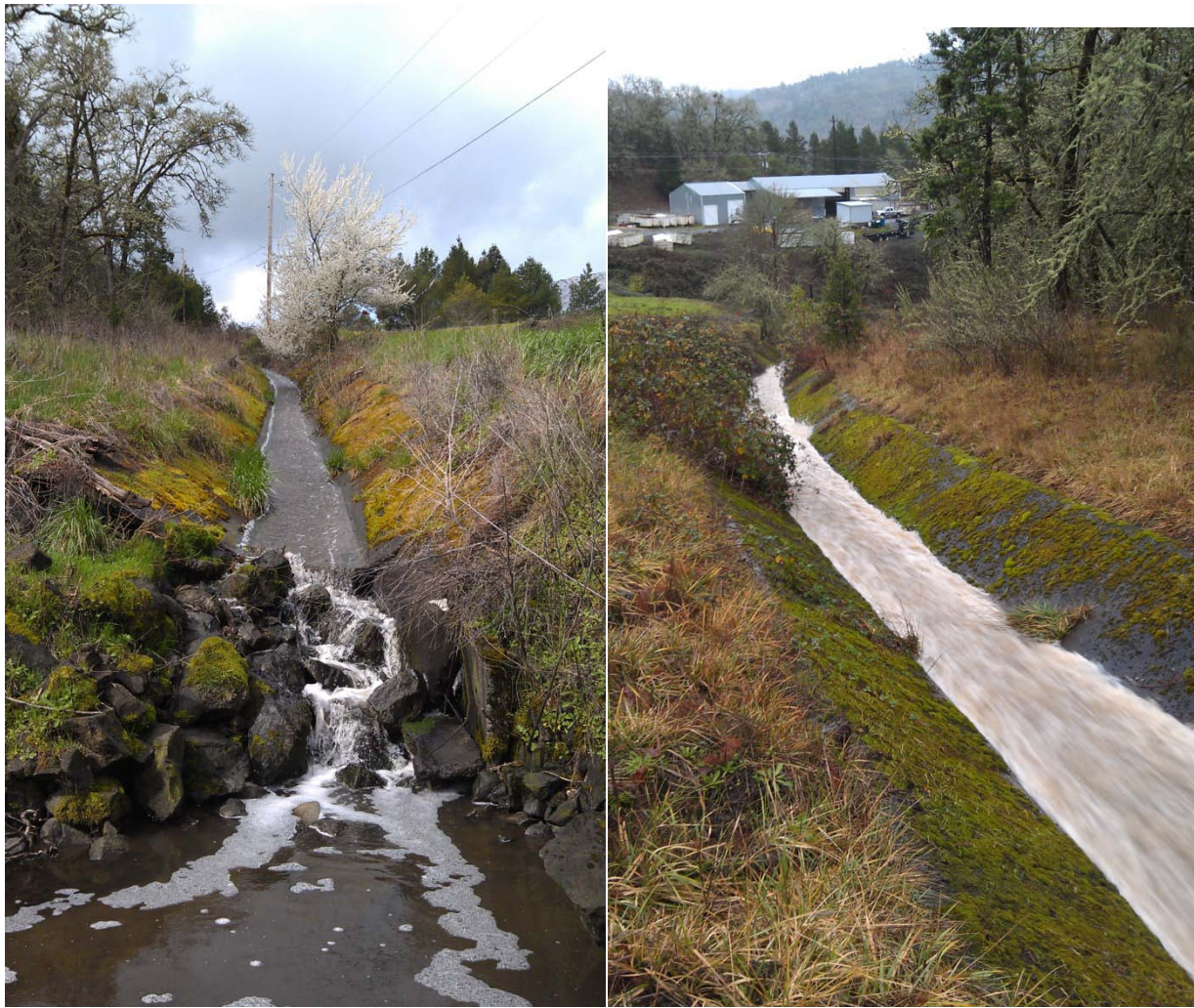
Figure 6. Concrete chute roughly 1,550ft up from the ODOT culvert.
