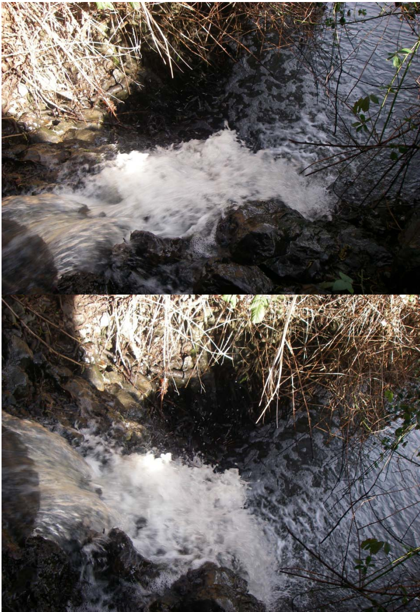
Figure 1. Approximate 10ft bedrock step at the end of the culvert.
